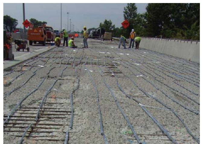
Galvanic anode system on bridge deck prior to placement of reinforced concrete overlay
