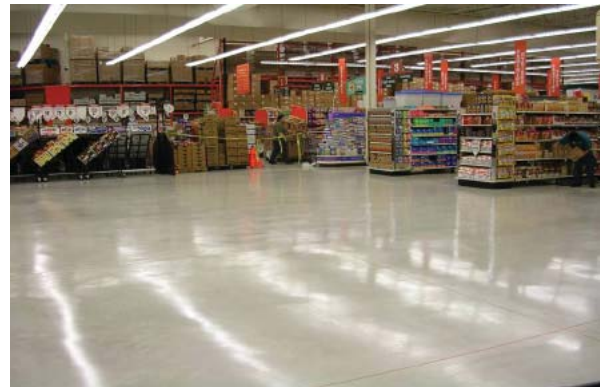
Typical steel trowel finished concrete with one coat of Durafloor HD and three coats of Durafloor HD-S.
