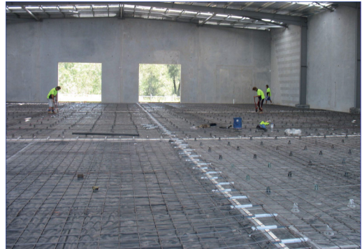
Square Dowel Cradles (with optional ground crack inducer under) set up prior to pouring concrete.
