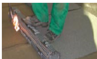
5. Torch lay the slate coated polymer-bitumen membrane facing upwards on Autotene Base
